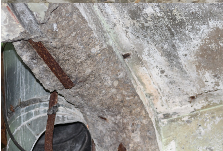
Photo 19 Damaged Floor Beam Area-C & D
