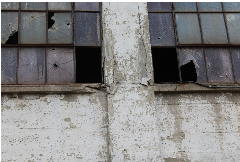
Photo 30 Column Deterioration - West Wall
