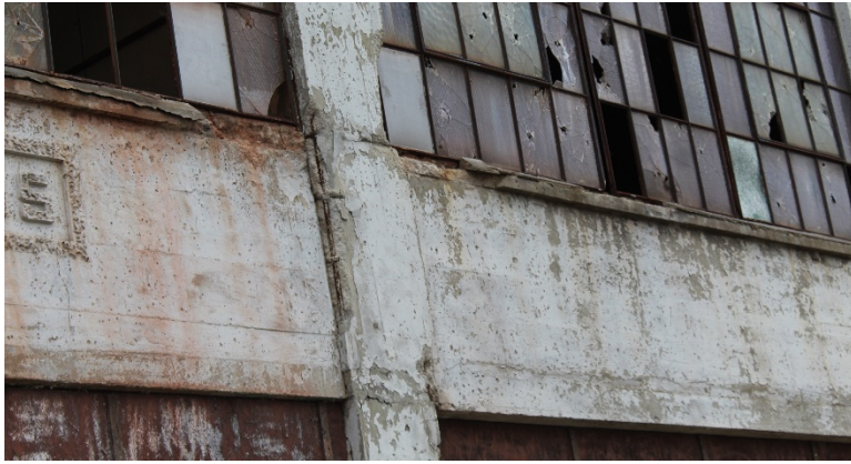
Photo 31 Column & Beam Connection Deterioration
