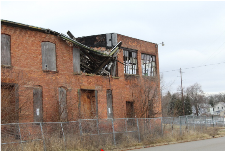
Photo 2 Area-A South Wall Roof & Wall Collapse
