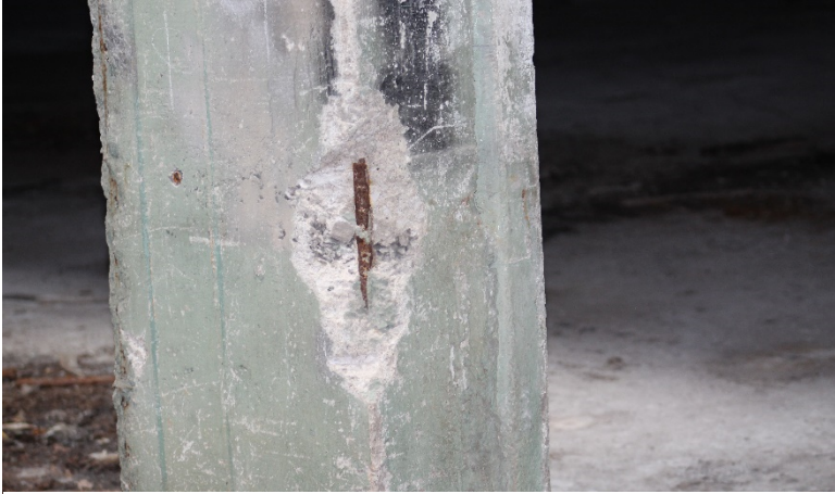
Photo 21 Exposed Column Reinforcing
