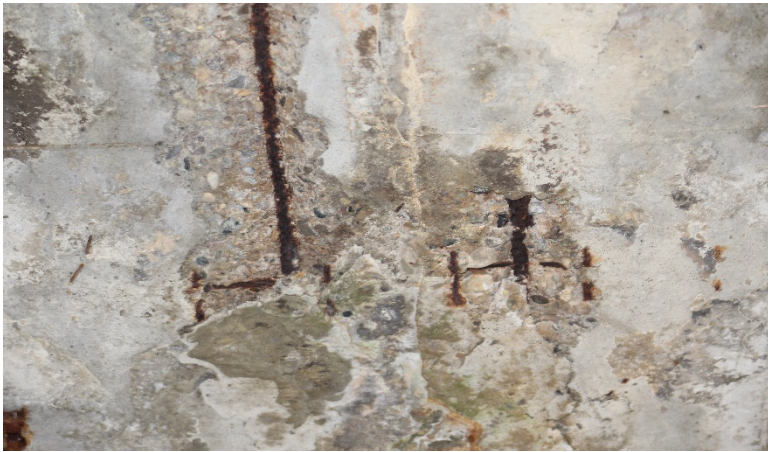
Photo 20 Exposed Floor Slab Reinforcing Steel
