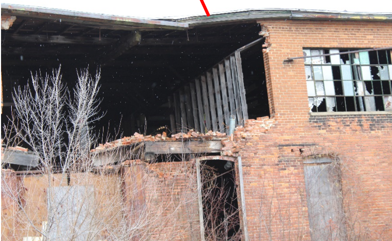
Photo 3 Area-A South Wall Collapse
