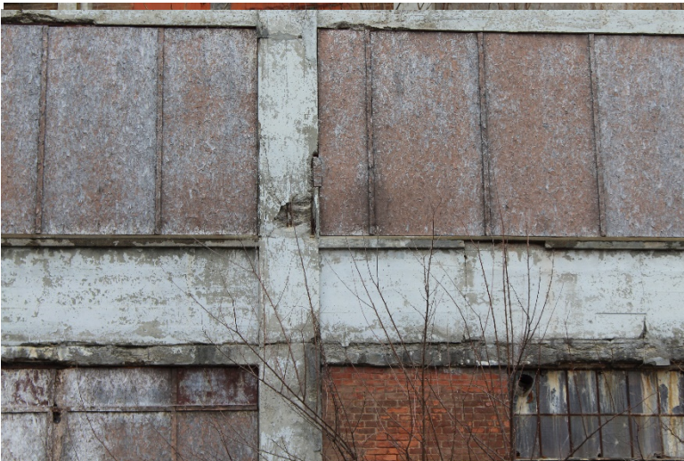
Photo 22 South Wall Deteriorated Column
