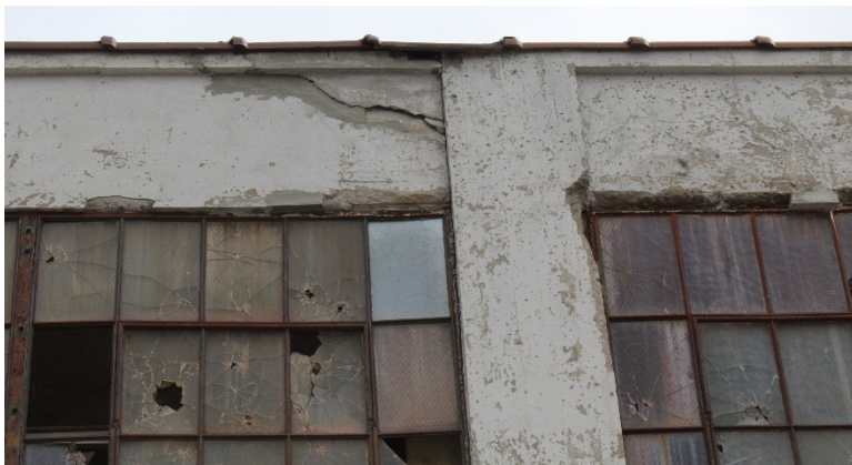
Photo 32 Roof Beam Damage w/ Failed Repair
