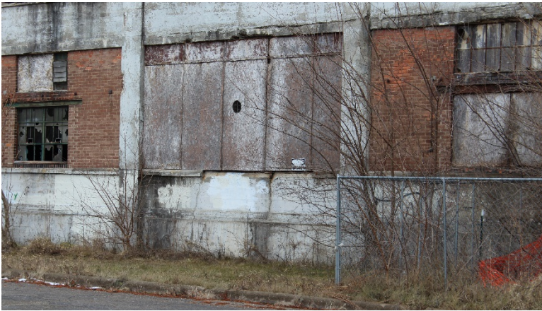
Photo 26 Exterior South Wall Ground Floor Cracked Beams
