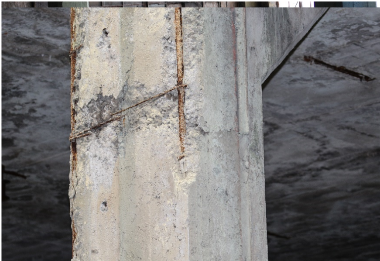
Photo 16 Exposed Column Reinforcing
