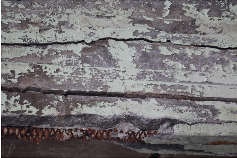
Photo 24 Several Cracked Roof Beam Area-D
