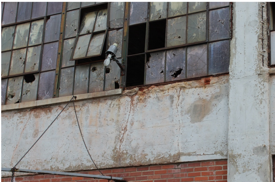
Photo 33 West Wall Floor Beam Cracking
