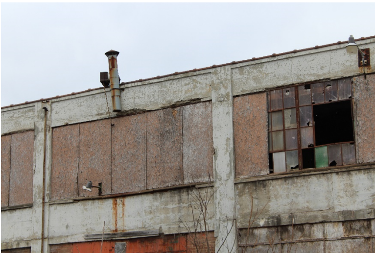
Photo 27 South Wall Area-D Structural Beam Cracking
